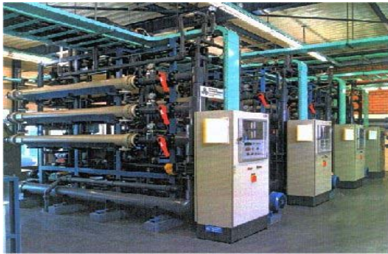
Micro filtration plant for recovery of acid in galvanizing plant
